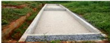
Constructed Wetland for Treatment
